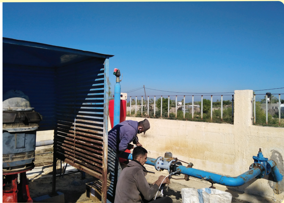
Local community workers installing components for the remote operation of Water Well.
