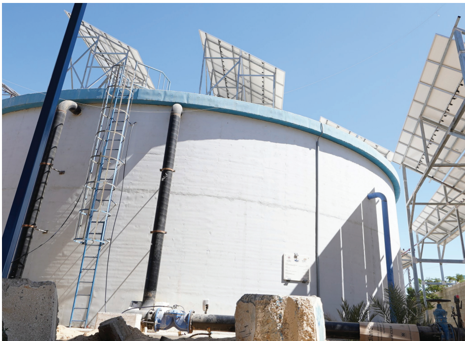
Canada Well, Rafah, Gaza. The ICRC has installed Solar PV, a net metering system, and a dedicated power line to support the Coastal Municipalities Water Utility in improving the operational resilience of the public water supply facility. Photo credit: ICRC
